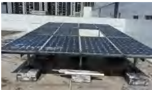
Figure 4-2 Rooftop Photovoltaics at Singapore Canadian International School
